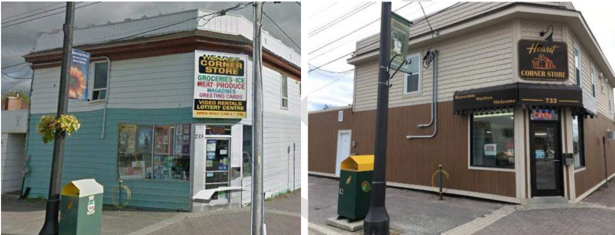
Figure 6-2 Example of before (left) and after (right) a façade improvement grant, Hearst, ON (Source - Google)
