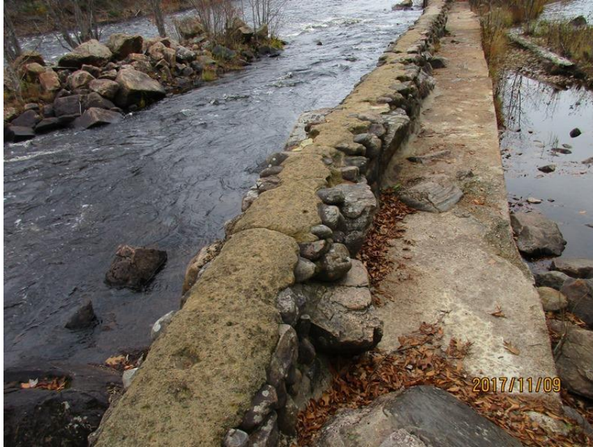
Rock Wall Walking Surface - and Trip and Fall Hazards
