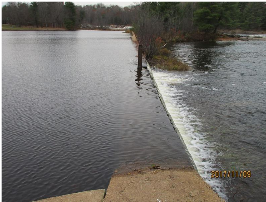
Outflow Wall – Looking North West (partially submerged structure)
